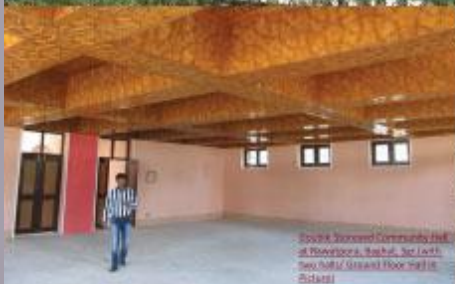
South Srinagar Community Hall at Patherpora, Srinagar. Top Left: Two halls at ground floor will be added.
